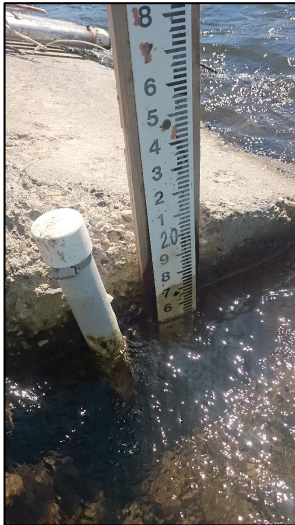
Figure 6. Typical equipment installed at monitoring sites that were visited quarterly for manual data download: a staff gauge and PVC stilling well with a suspended pressure transducer.
